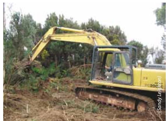
A modified root rake on an excavator (“the claw”) was used to grub gorse
